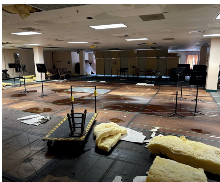
The Peterson Great Room, second floor of the Pavilion, after Hurricane Milton.
